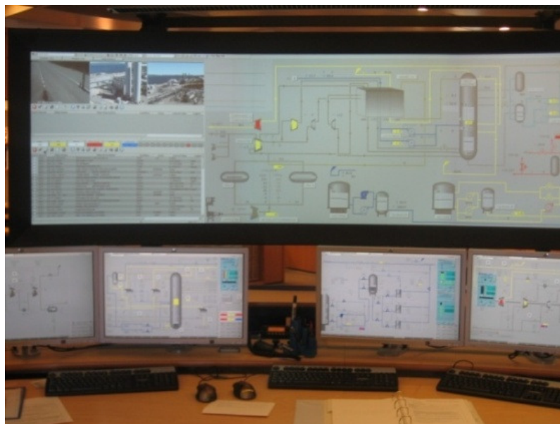
Figure 3. A control station.
