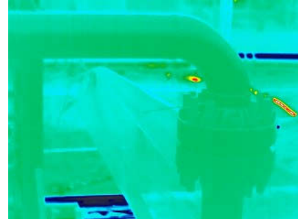
Fig. 5. Thermal pictures of the pipe.
